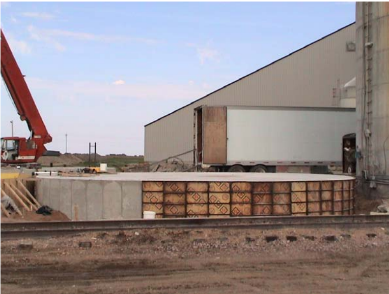
New dryer pad was poured on May 13, 2005. This pad contains over 82 yards of new concrete poured over and around the old silo pad.
