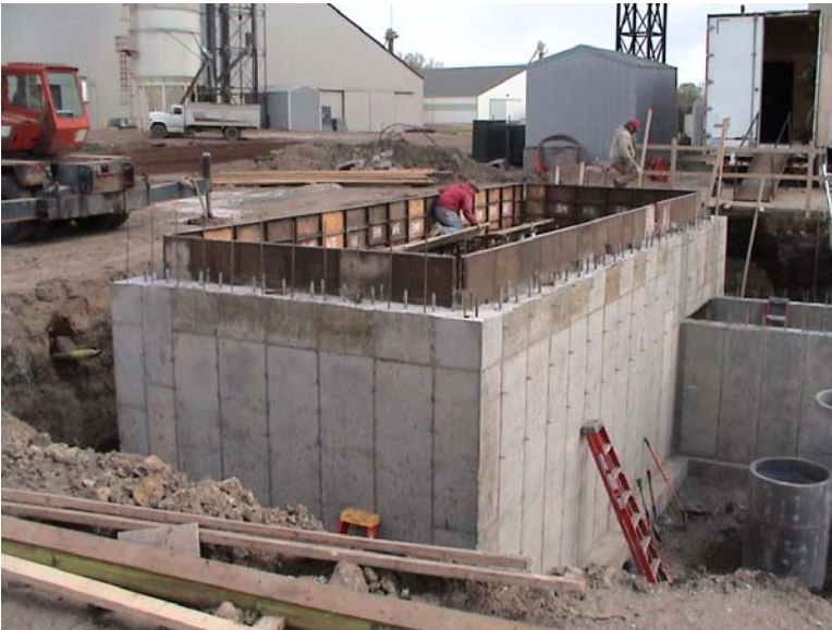
This will be the new dump pit, it will be large enough to pull on a semi and dump both hoppers without pulling forward. Rated capacity will be 17,500 bph.
