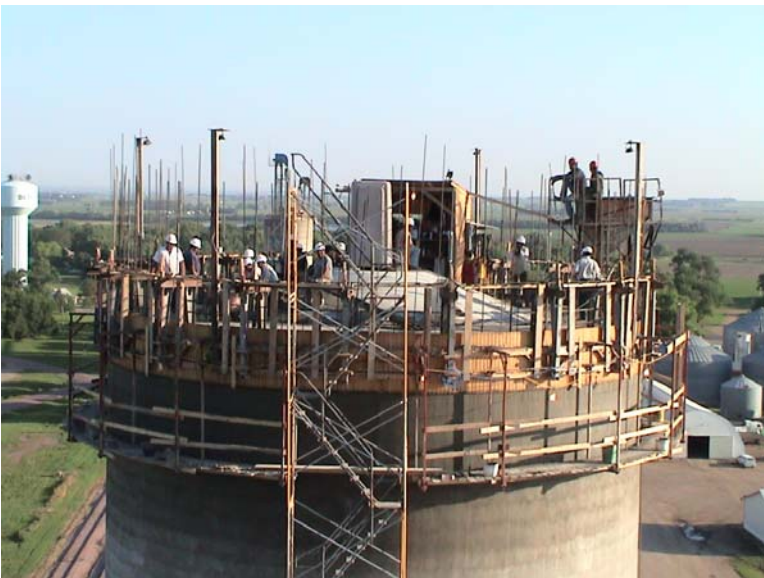
Top of the slip at 7:30 a.m. Friday Morning. The pour has went so well that they should be done by 7:00 p.m. this evening.
