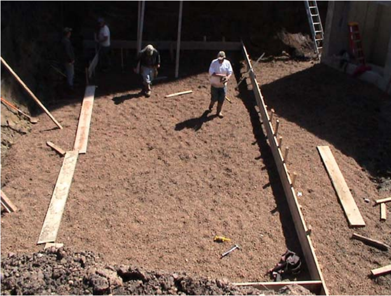
Photo taken on April 13 th of forming for new dump pit floor.
