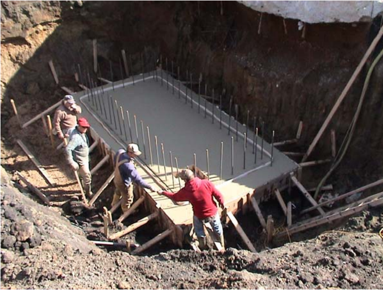
This is the floor for the new boot pit which was poured on March 31 st .
