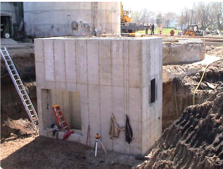
This is the boot pit. This will hold the boot of the 17,500 bu/hour leg which will feed both wet silo and new dryer. This pit will have drainage tile buried around it and will be wrapped in bentonite board for waterproofing.
