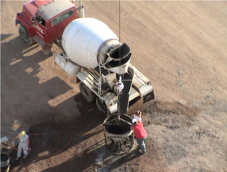
Picture showing the crew and concrete truck ready to fill bucket trip up to the top.
