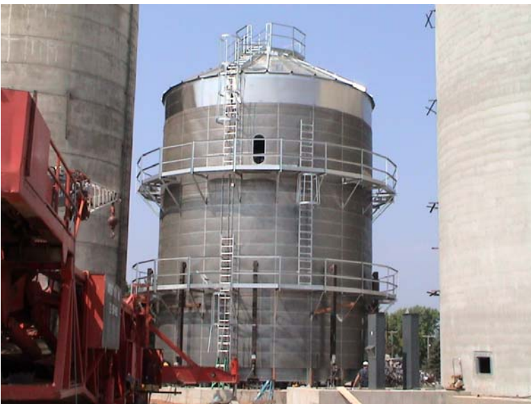
Picture of new dryer under construction. Picture taken the morning of July 11, 2005.
