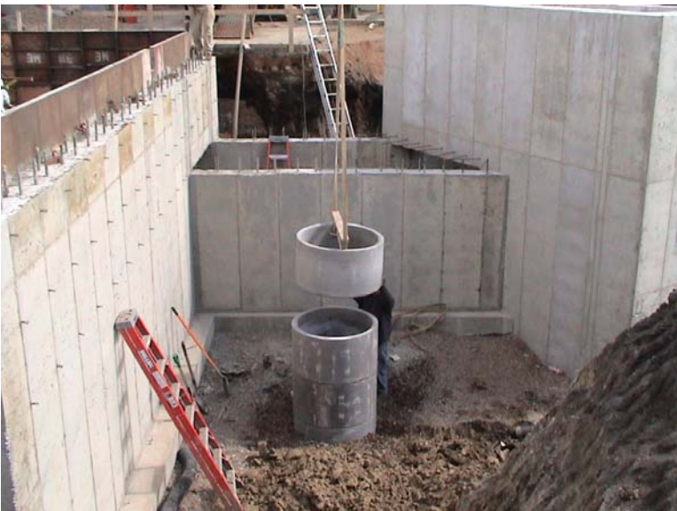
Construction Crew is setting well casings for sump well. Both the dump pit and boot pit are tiled around and directed to the sump well.
