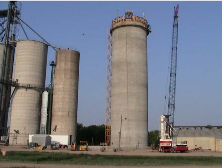
Silo slip was finished at 5:30 p.m. Friday the 17 th of June. Final silo height was 140 feet making it the tallest silo. The slip total time it took for the pour was 105 ½ hours for an average of 15.92 inches per hour.
