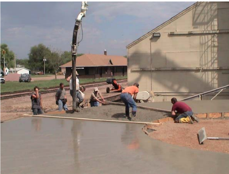
Crew finishing pouring of silo foundation. The donut foundation of the silo is 15 foot wide and 3 foot deep. The foundation took 4 hours to pour and 200 yards of concrete.
