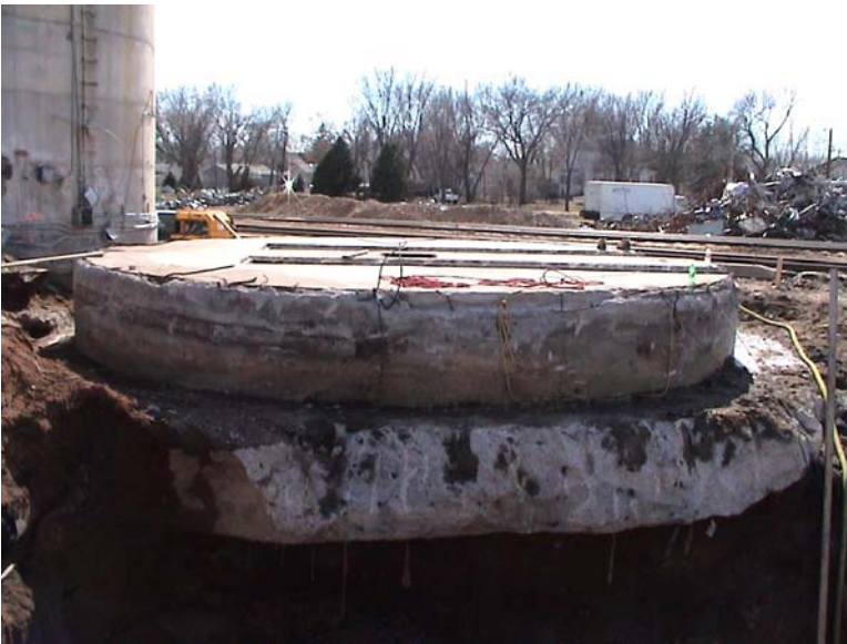
This is the old silo foundation. Nohr Engineering of Yankton has approved this for as a foundation for the new 10,000 bu/hour Zimmerman Tower Dryer. They will pour a 1 foot outside wall completely around the old foundation and a 1 foot cap over the top of foundation with rebar doveled back into the existing foundation. Photo taken on March 31 st .
