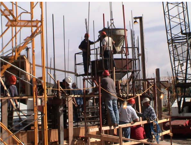
Picture of crew working on slipform pour early Monday, June 13 th . They will pour 24 hours around the clock with 2 crews working 12 hour shifts.
