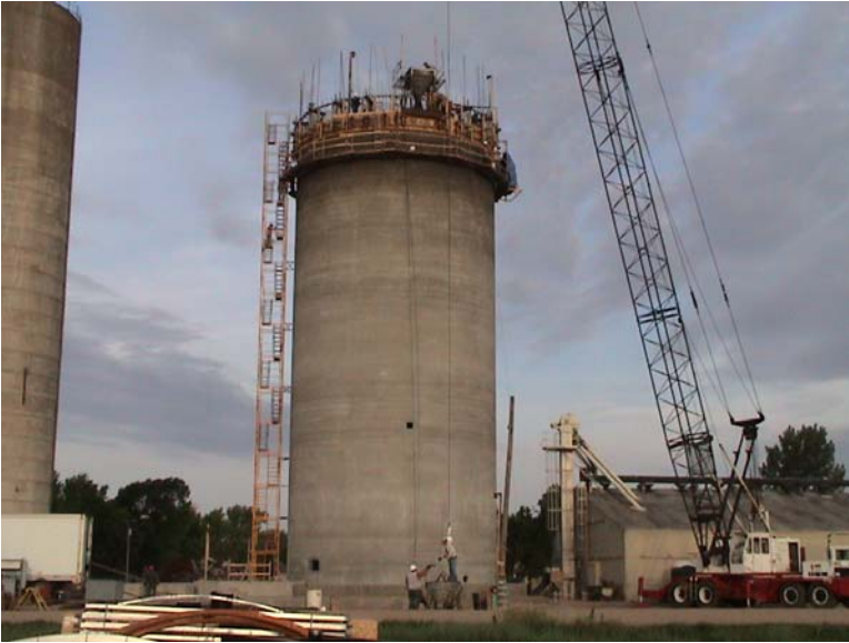
Picture of slip taken Thursday morning. Slip was at 90 feet.
